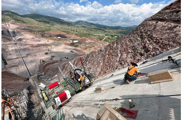
Grouting on the east abutment at Chimney Hollow Reservoir took place on 45-degree angles.
